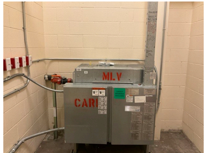
28 - ELEVATOR CONTROL ROOM
