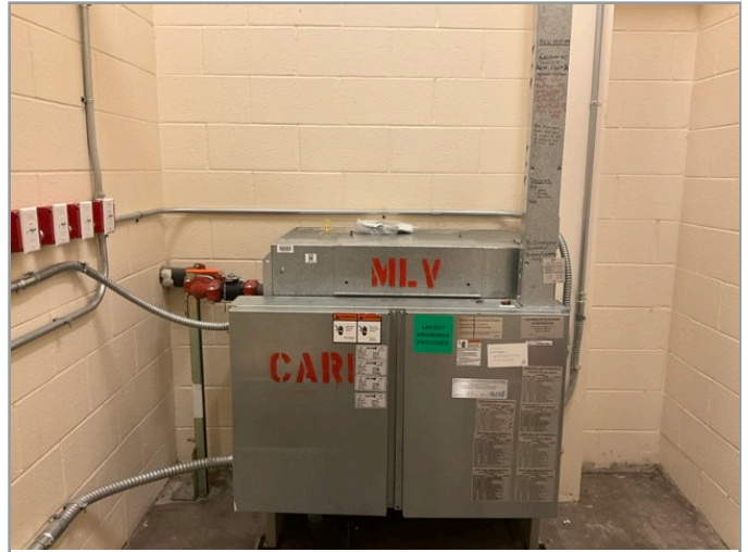
ELEVATOR CONTROL ROOM
