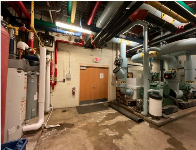
21 - MAIN MECHANICAL ROOM
