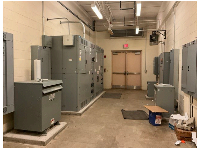
22 - MAIN ELECTRICAL ROOM
