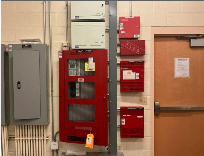
25 - FIRE ALARM PANEL
