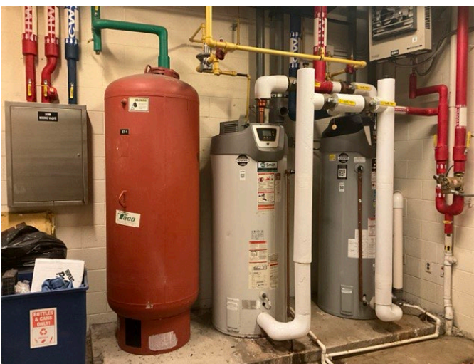
23 - DOMESTIC WATER HEATERS
